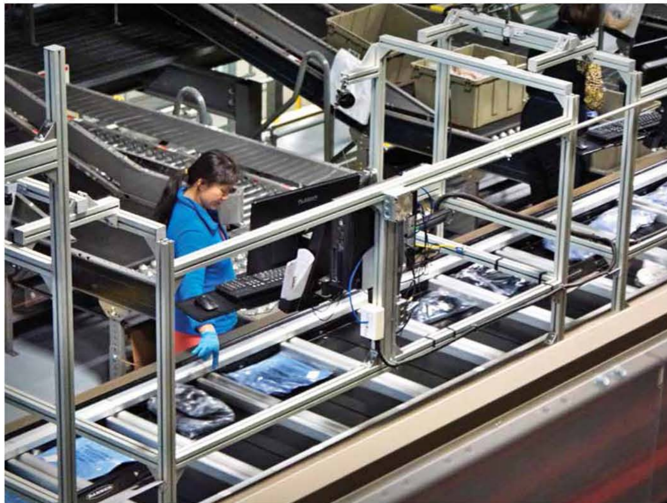
The heart of the facility is a bomb-bay unit sorter that feeds 600 chutes and processes 15,000 units an hour. The sorter manages store fulfillment, wholesale distribution and online fulfillment.
